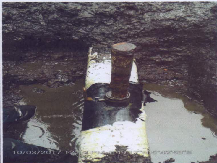
B: LEAK POINT AFTER OPENING AND PEGGING
